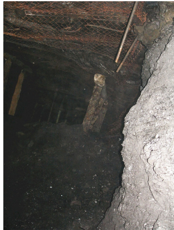
Fig. 1 Coal burst in the Kailuan Qianjiaying coal mine
