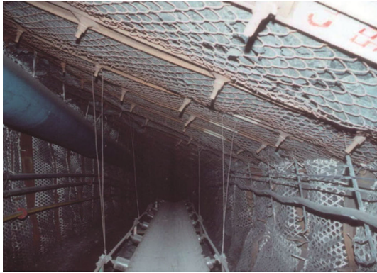
Fig. 7 Profile of bolted maingate with depth over 1,000 m in Xinwen coal mining district
