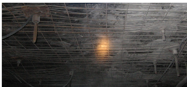
Fig. 7 Meshed roof in the trial roadway
