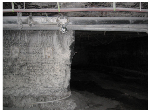
Fig. 6 Cluttered rib wall and cut-through
