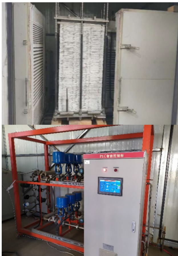
Fig. 4 20 kW MCFC single stack
