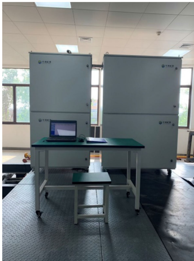
Fig. 3 10 kW SOFC system
