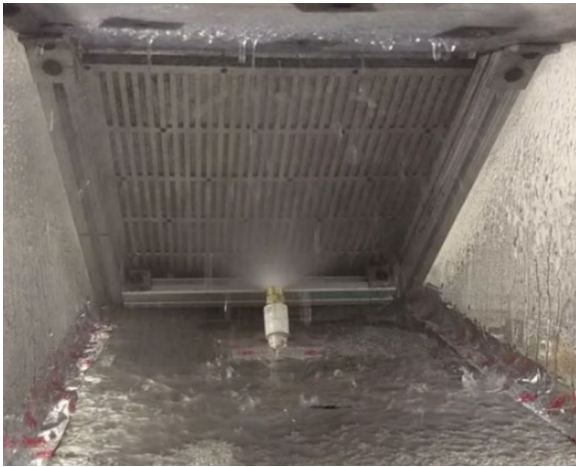
Fig. 7 Filter installed in the duct
