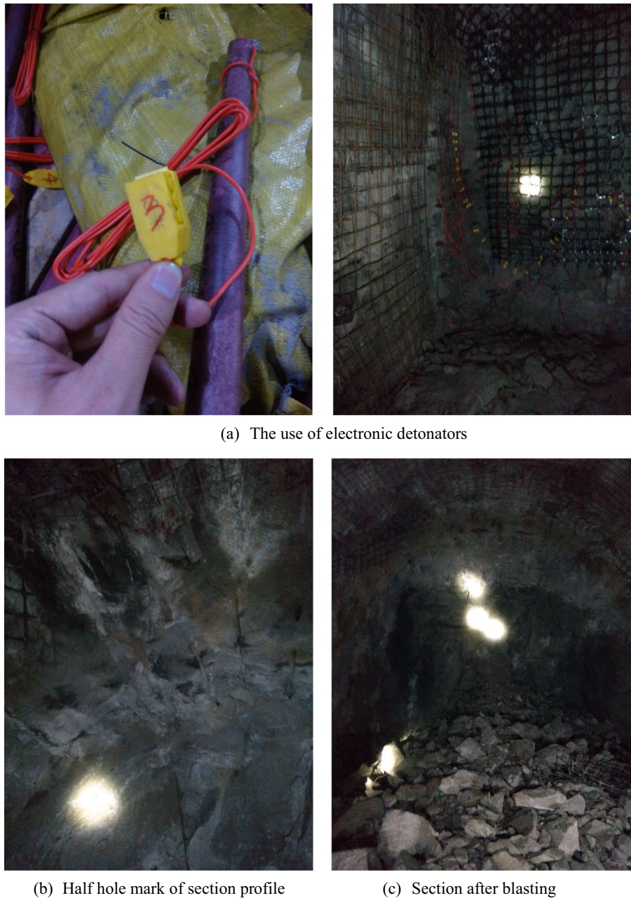
Fig. 22 Drilling and blasting process of on-site working face. a Setting time of digital electronic detonator; b Half hole mark of section profile; c Section after blasting
