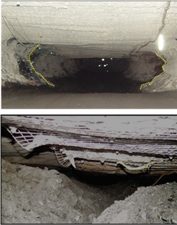
Fig. 1 Effect of a coal burst on roadway (the top shows the roadway before the burst, and the bottom is after the burst)
